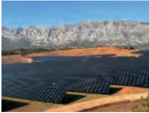
Owner of 6.5 MWp solar power plant in the South of France, near the village of Puylobrier since 2011 (First Solar modules)
